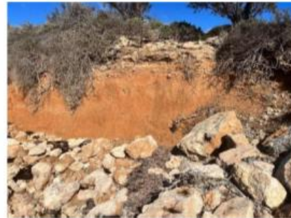
Figure A7: Erosion fronting car park
