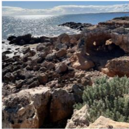
Figure A32: Showing southern side of breakwater and erosion impacts to Point Warrene
