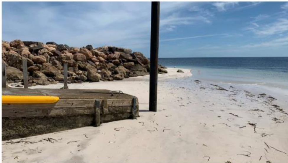
Figure 4: Sediment accumulation at toe of the boat ramp (Progress Association March 2021)
