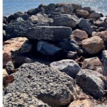
Figure A27: Northern extent of breakwater showing poor condition
