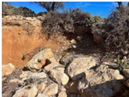
Figure A8: Erosion pinch point fronting car park (2m from edge of car park)
