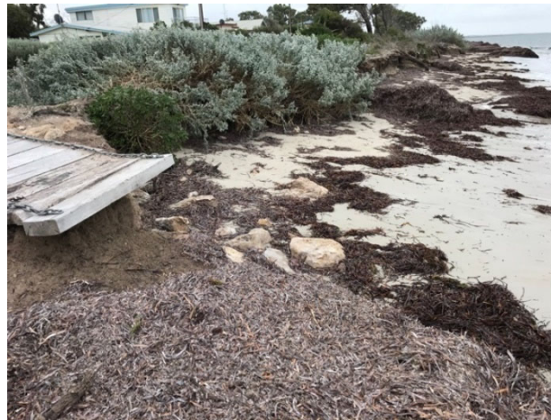
Figure c: Access way to beach in front of 9 Mud Alley where ~5m of recession has occurred since 2019.
