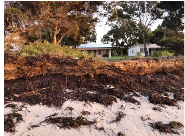
Figure d: Recently impacted erosion escarpment is observed along most of Mud Alley.
