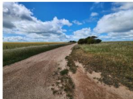
Johns Road at improvements on Section BE looking south east toward intersection
